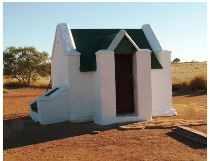
The cellar at Tennant Creek telegraph station before and after recent conservation work.
